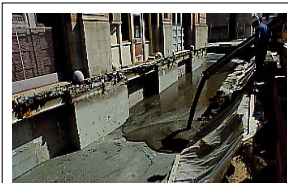
Figure 5-15: CLSM being placed in lifts to manage the load on basement walls.
