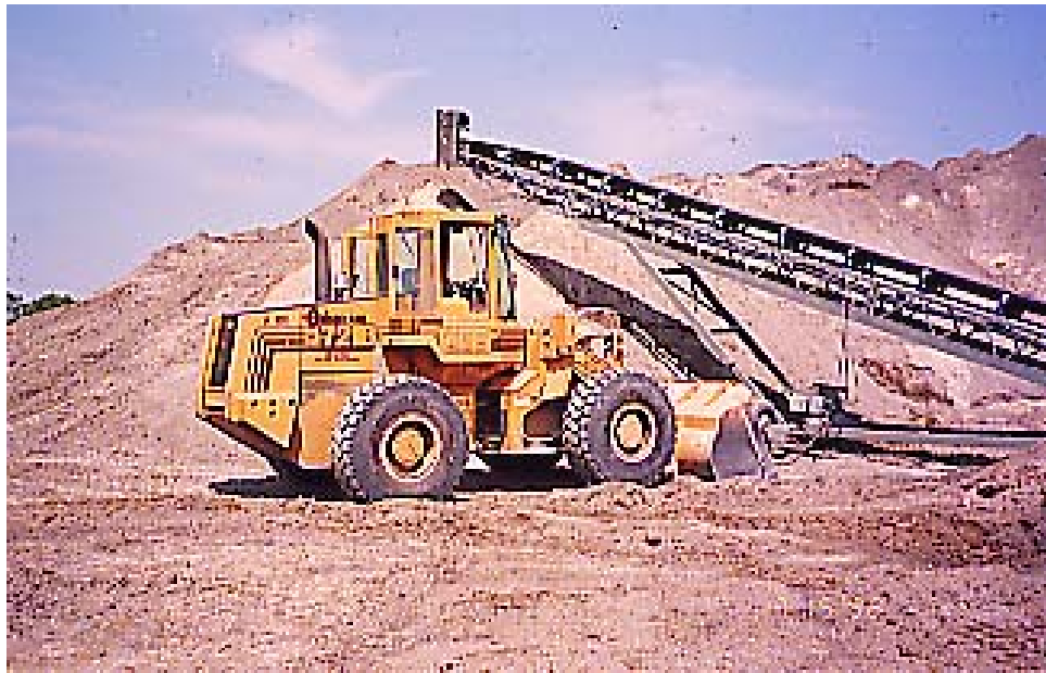
Figure 6-9: Coal ash recovery from the Pleasant Prairie Power Plant ash landfill for use as granular base course material
