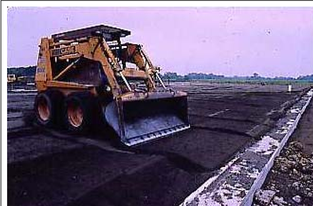
Figure 6-4: Bottom ash structural backfill being used for building construction in Racine, Wisconsin
